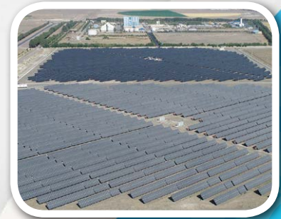
■ solar power plants number 1 and 2
